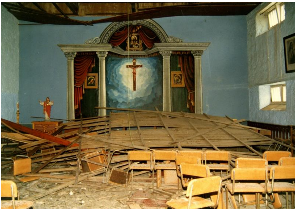
1999.749.9 Image documenting the damage in the Catholic Chapel following the 1988 riot
