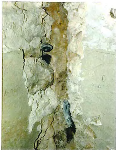
Plate 16. Lead pipes, Cell B37
