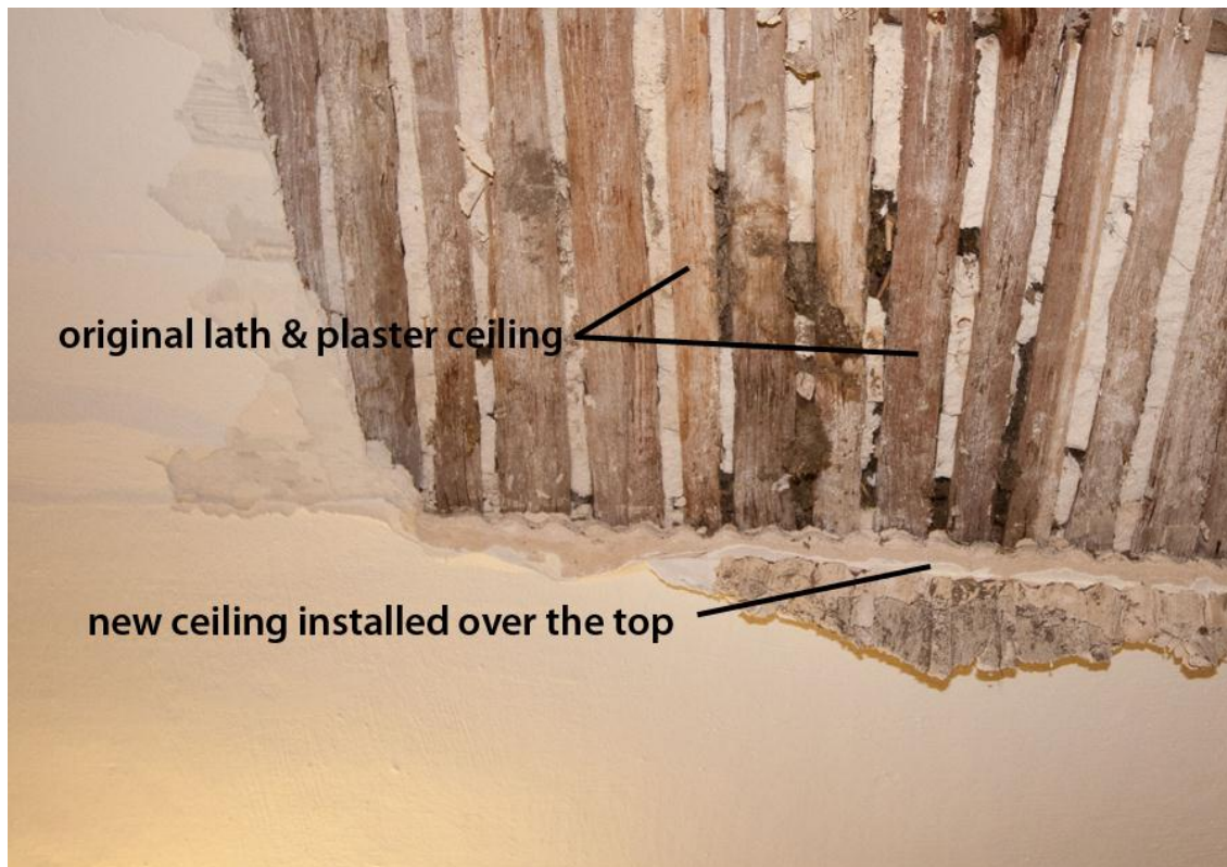
Figure 5.1: Collapsed ceiling in cell D66 showing stratification. Photograph by E Mein, 2012.
