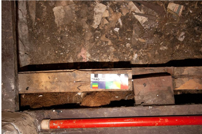
Joist space 4 with mouse nest prior to removal
