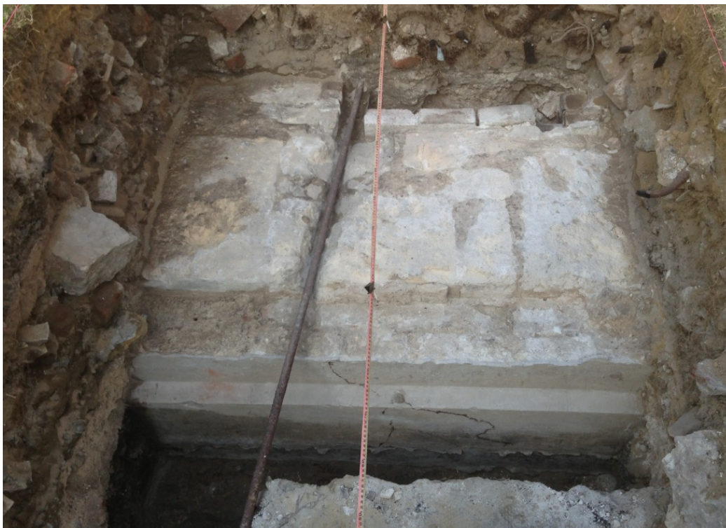
Figure 16: Chimney structure, with the brick extension and concrete render shown around the limestone core.
