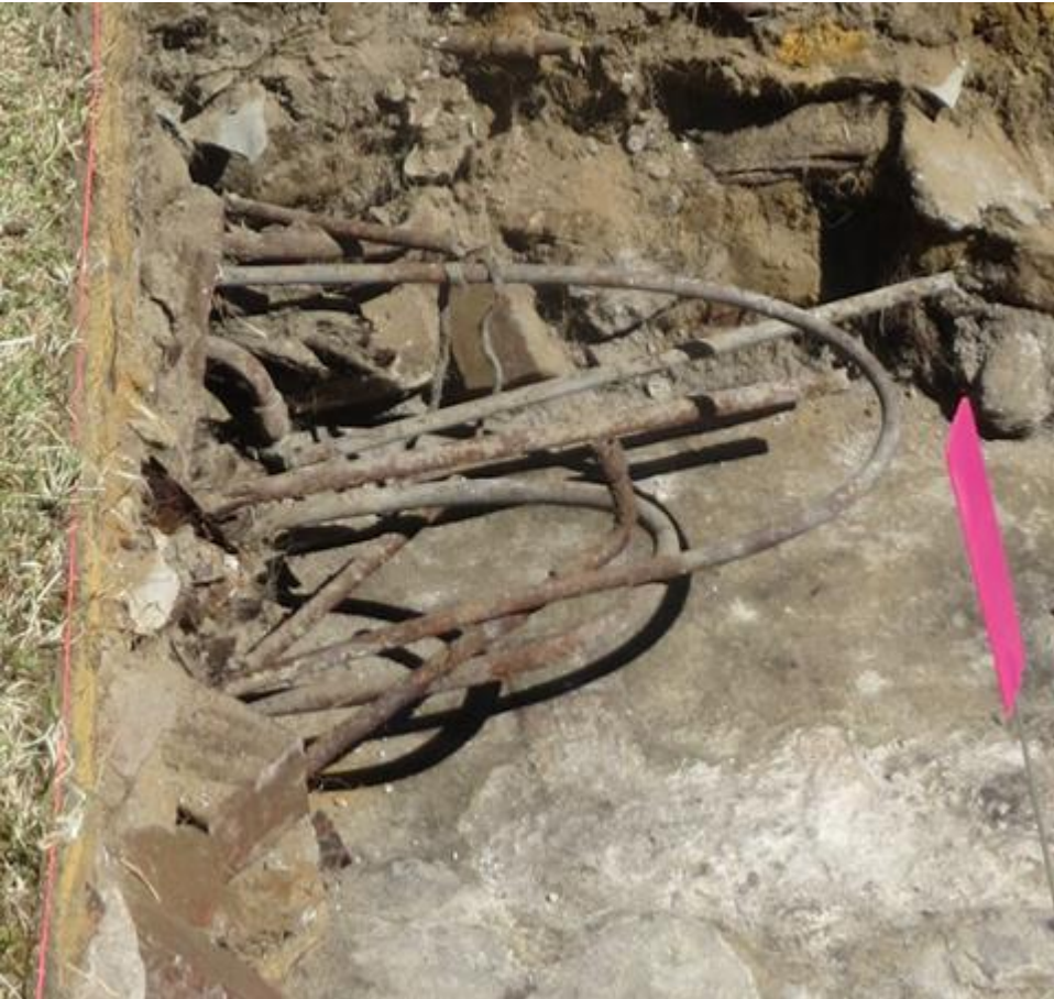
Figure 5: Piping in Trench 1.
