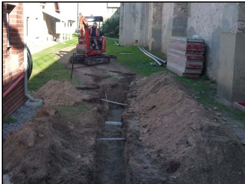
Plate 2: View of trenching works in the Northern Courtyard of the Female Division
