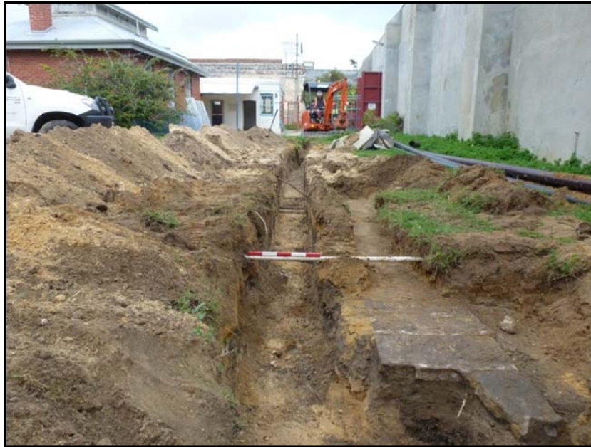
Plate 15: View of realignment of Trench ST12 (note flagstone path C.93), looking south (Scale = 50 cm)
